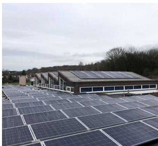
7. Chesham Primary School, Bury (49.68 kWp)
