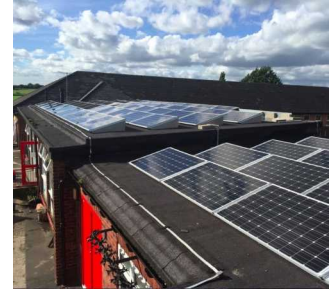
3. Irlam Primary School, Irlam (28.62 kWp)
