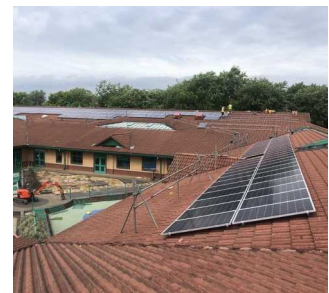
9. Springwood Primary School, Swinton (49.68 kWp)
