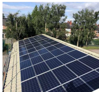
8. Monton Green Primary School, Monton (29.7 kWp)
