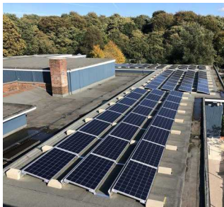
4. Peel Hall Primary School, Little Hulton (49.68 kWp)
