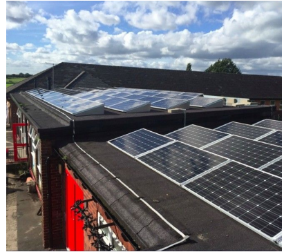
3. Irlam Primary School, Irlam (28.62 kWp)
