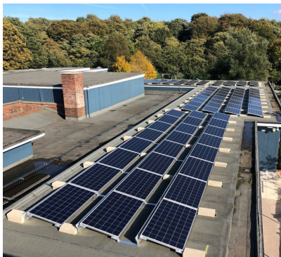
4. Peel Hall Primary School, Little Hulton (49.68 kWp)
